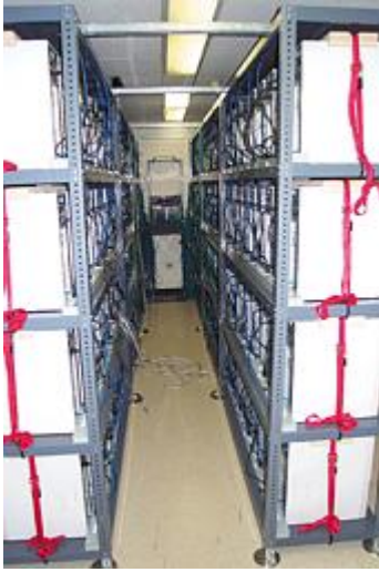
Figure 3. 156 Dual-Processor PC Cluster. The boxes are connected using a standard 100Mbps Fast Ethernet network (the green and blue cables). In the back, one can see the 192-port Cisco switch. The height of the shelving system is approximately eight feet.
